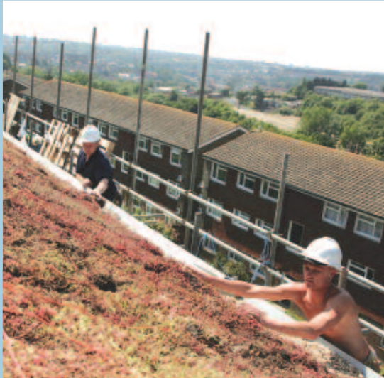
Laying the sedum roof of The Bridge community centre at Ore Valley, Hastings Millennium Community
